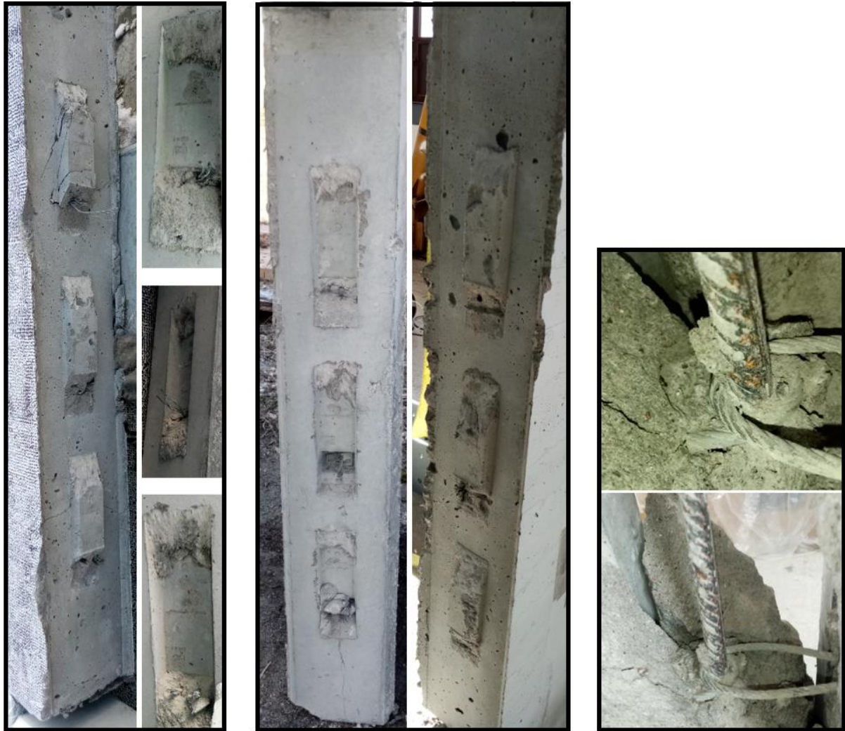
Figure 4-18 WL2 specimens after testing (from left to right: 1 st test, 2 nd test, 3 rd test)
