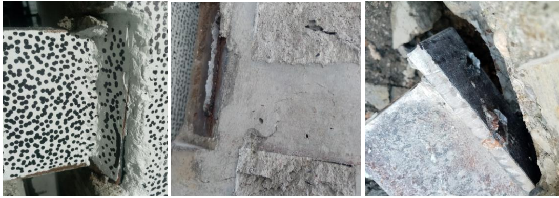
Figure 3-20 Indications of embedded insert pullout (from left to right) SA2T1, SA2T2, SA2T3 (anchor welds failure)
