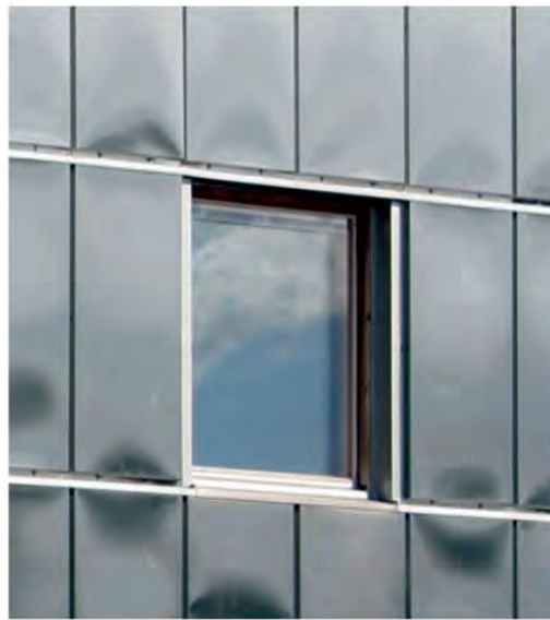
Figure 8.2: Austenitic stainless façade which has buckled under intense sunlight. Unless this is desired as an architectural feature, a duplex or ferritic grade with lower thermal expansion may be preferred.
