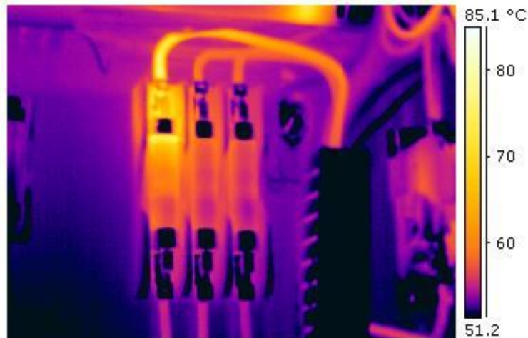
Fig. 6.6. Infrared thermograph showing hot electrical equipment[25]
