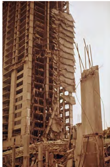
Figura 11. Eșecul The skyline plaza apartment BUILDING
